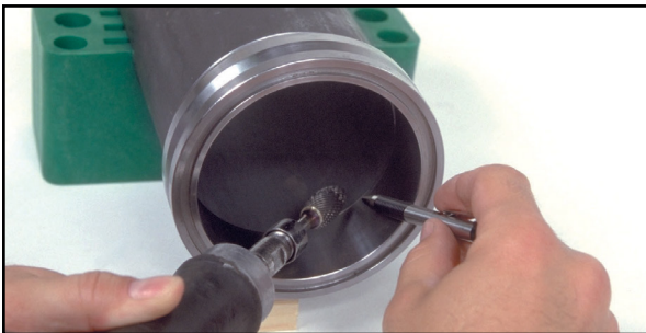
Step 3: Grind the weld on the inside of the pipe using a pencil type grinder. Clean the inside of the pipe after grinding.
